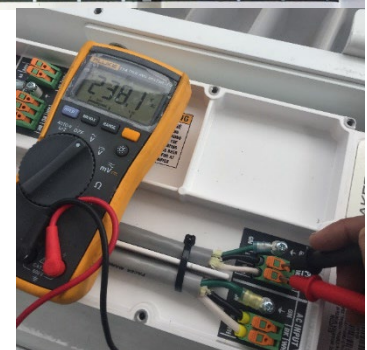
Testing SW Pump voltage
