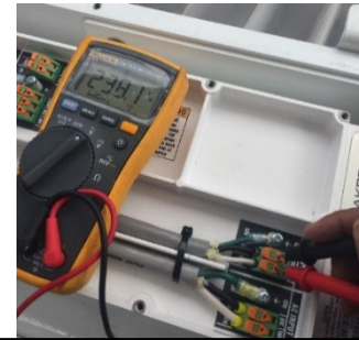
Testing SW Pump voltage
