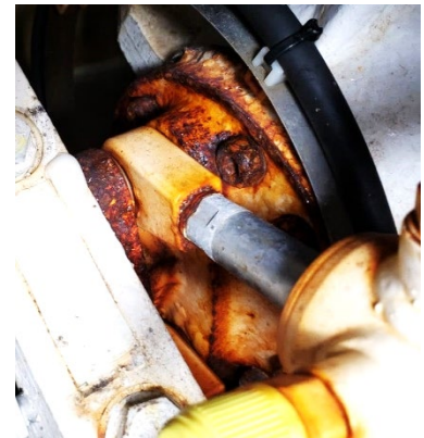
Seakeeper 3 with severe corrosion at rod end clevises, pins, and gimbal shafts
