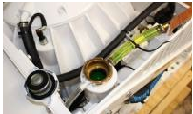
Glycol flow may be seen through fill cap
