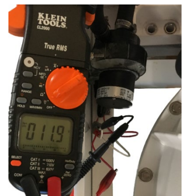
Image of technician back probing glycol pump connector for voltage
